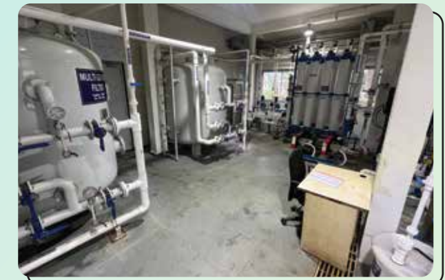
Secondary ETP RO Treatment plant at ETB-Pithampur
